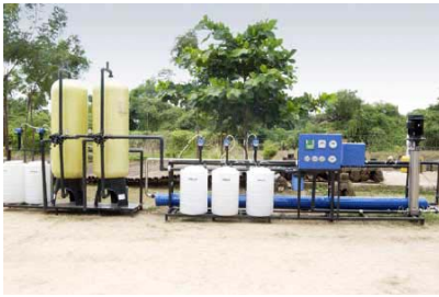
Figure 7: Small-scale reverse osmosis technology
