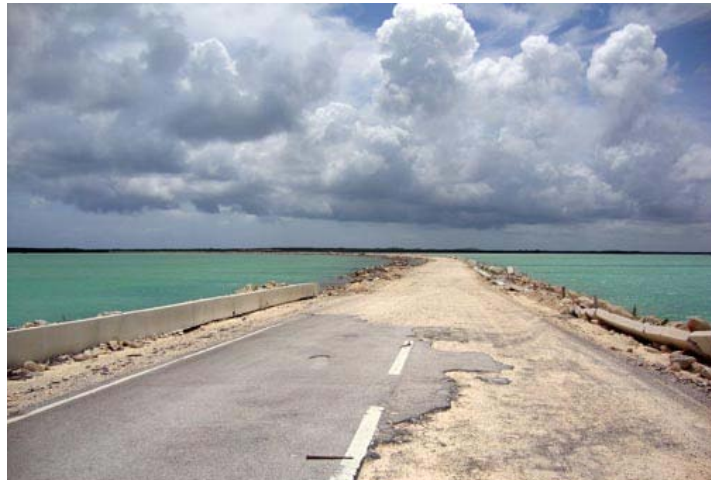
Figure 8: Damaged causeway connecting Middle and North Caicos following Hurricane Ike, 2008
